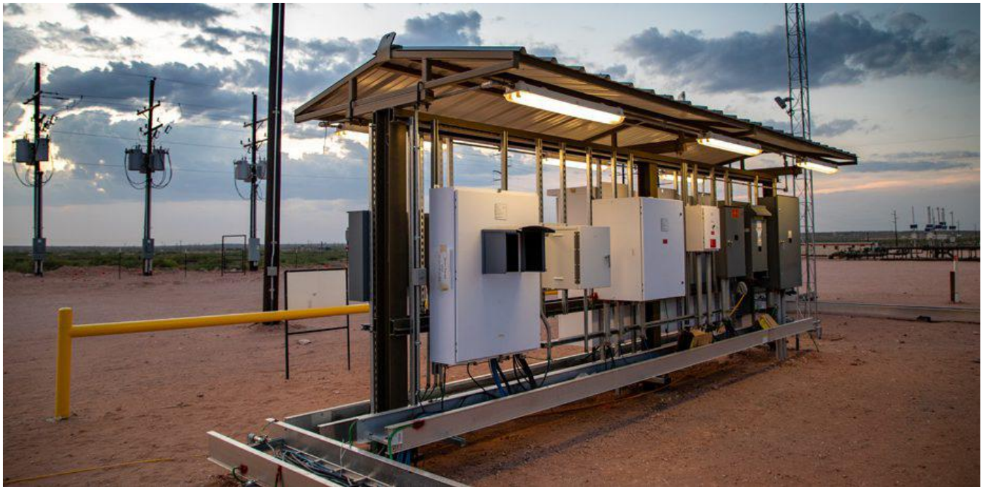
Command station for automation equipment at a facility in the Delaware Basin.
