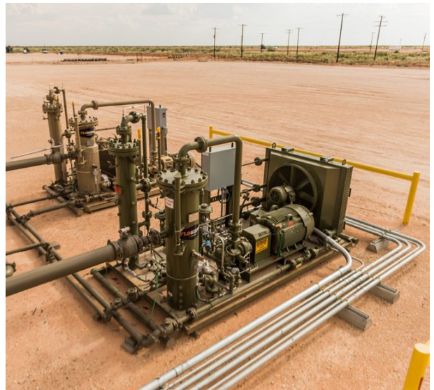
Vapor recovery equipment — Delaware Basin
