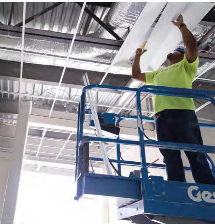
▲ New construction projects across the city require skilled workers. A master electrician's apprentice installs lighting in the New Center neighborhood.
