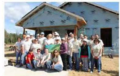
Entergy Texas’ Volunteer Council’s western region teamed up with the Montgomery County Habitat for Humanity to help build a home in Conroe for a family in need.
