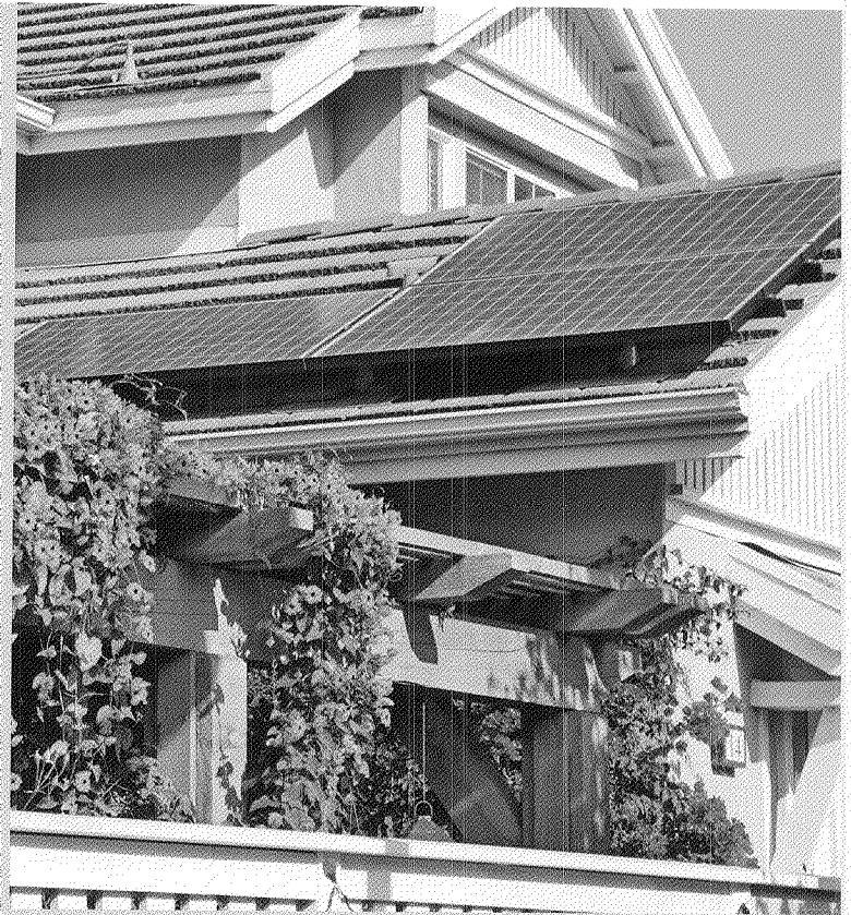
Enabling Distributed Energy: Southern California Edison has been helping customers put solar power generators on their rooftops for many years. These photovoltaic solar panels are on an SCE customer's home in Irvine, Calif.
