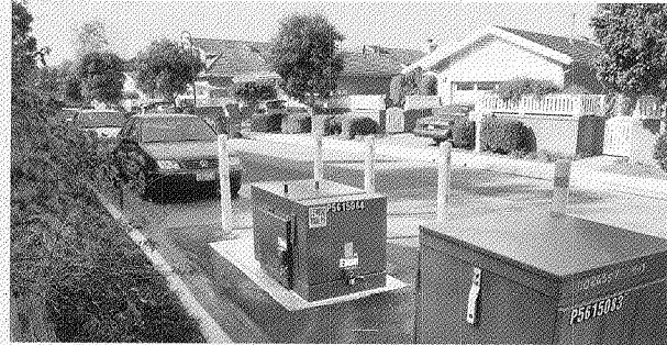
Storing Energy Locally: Batteries can be used locally in homes and neighborhoods to store energy from customers' distributed generators, such as in this neighborhood in Irvine where these transformers sit atop underground batteries.
