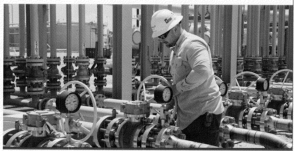
Operator at Hastings EOR facility
