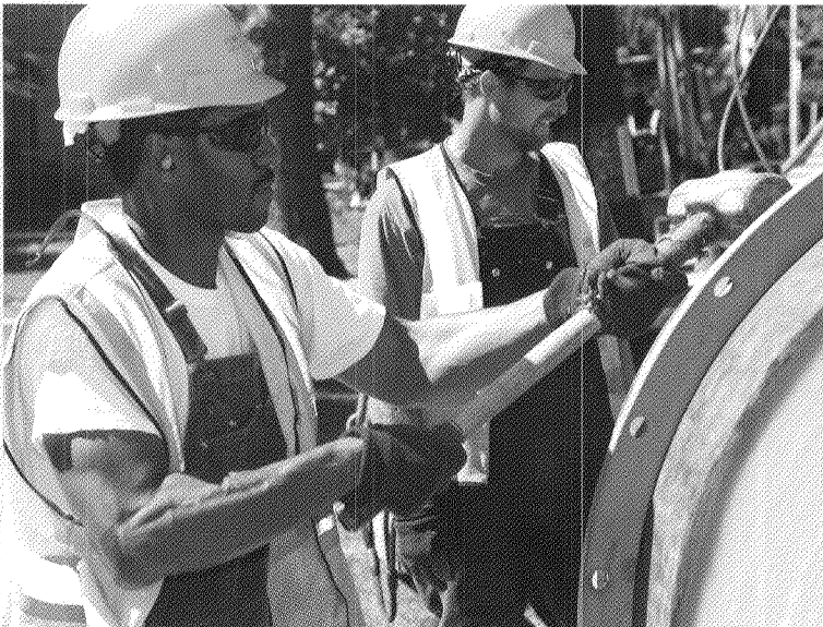
Below: From left, Damien Fowler, Gas Mechanic, and Dave Ahlgrim, Operations Apprentice, both with Peoples Gas
