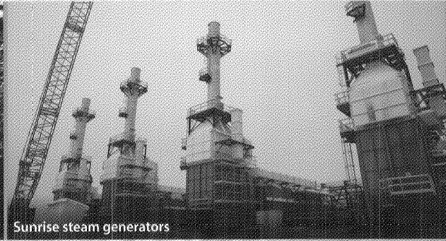
Sunrise steam generators
