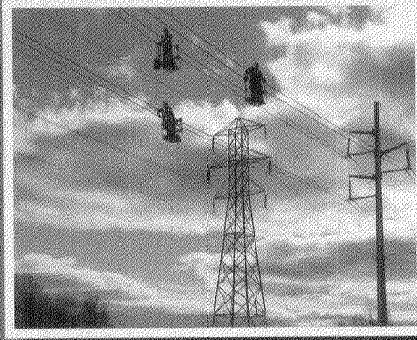
33 miles of new 115kV transmission line and 4.2 miles of 115kV rebuild for the Spier Falls to Rotterdam project is currently under construction in New York for National Grid.
