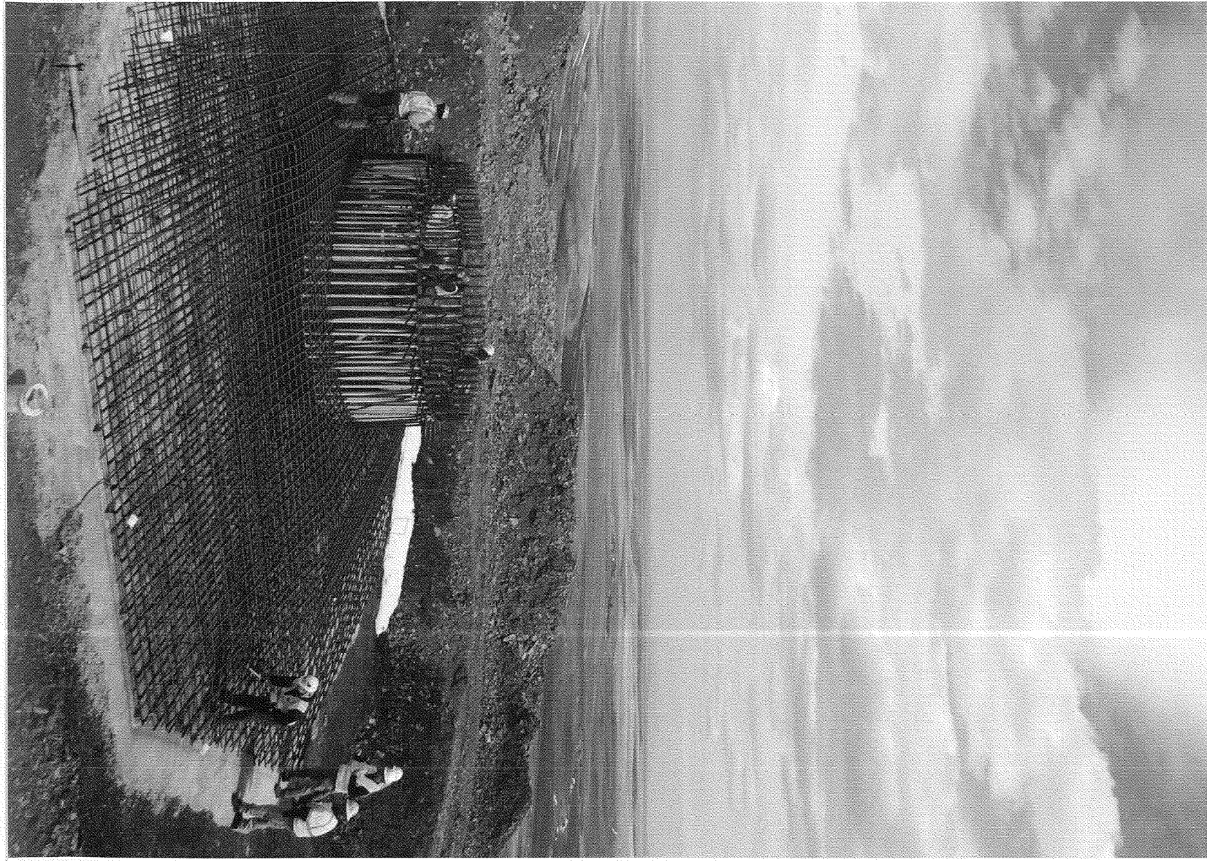
Contractors install up to 20 tons of rebar into footings for a single turbine at the company's Spion Kop wind farm.
