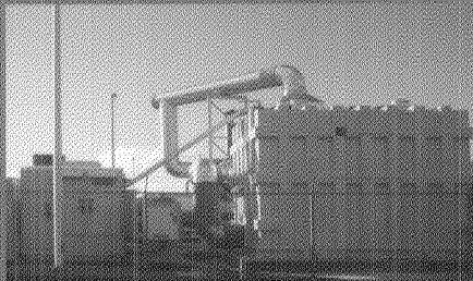
1.4 MW DFC1500 Wastewater treatment facility - California, USA
