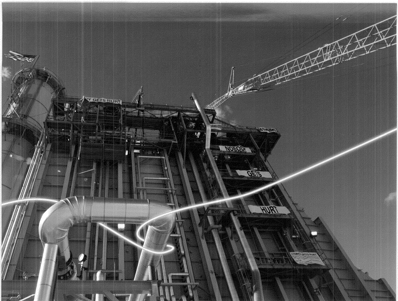
Langley Gulch Power Plant
