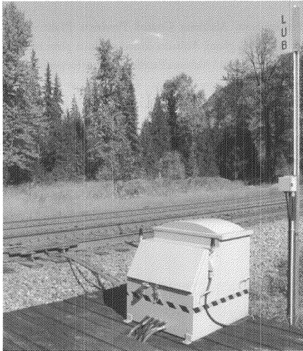
Remote notification activates PROTECTOR rail lubricator to apply friction modifier to track
