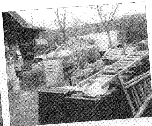
Only the garden took back stage due to all the building materials.
