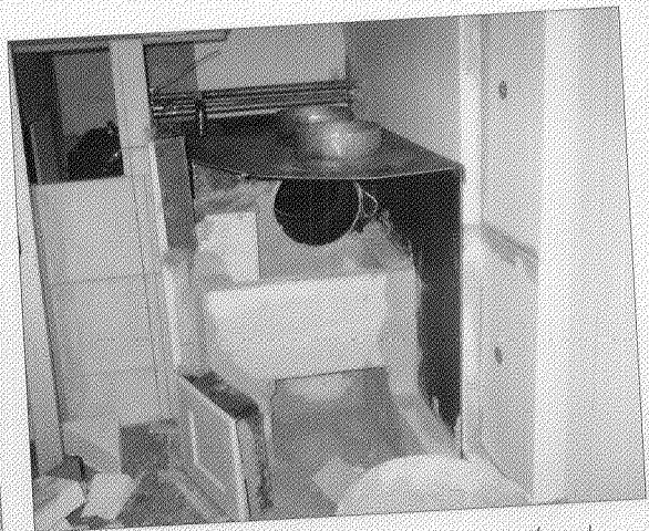
2007: hardly any energy costs thanks to the new house front and stove.
