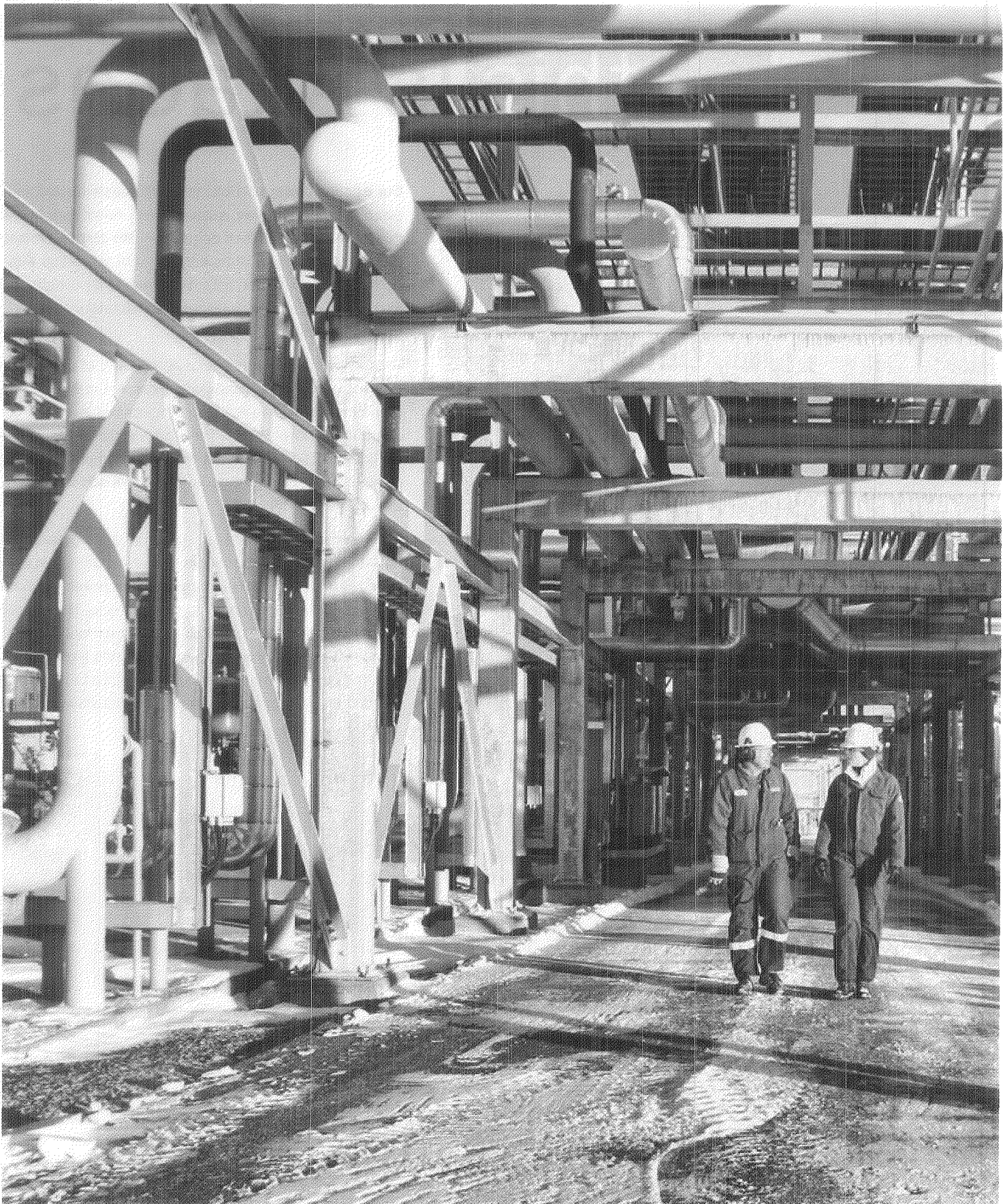
Solvent extraction facility, Alberta
