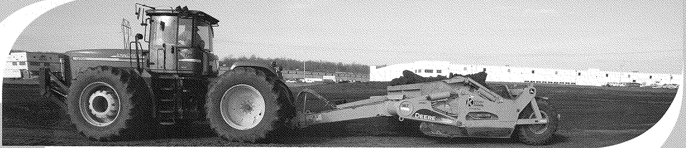
Ground clearing commenced in December 2009. Despite one of the worst winters on record, the project remains on schedule.
