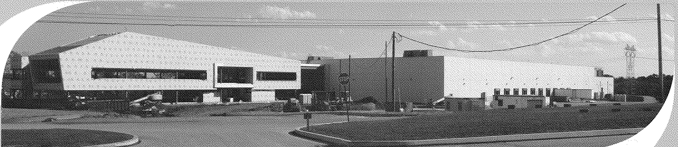
By September 2010, construction of all external sections of the facility had been completed.
