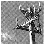
Base Station Infrastructure
