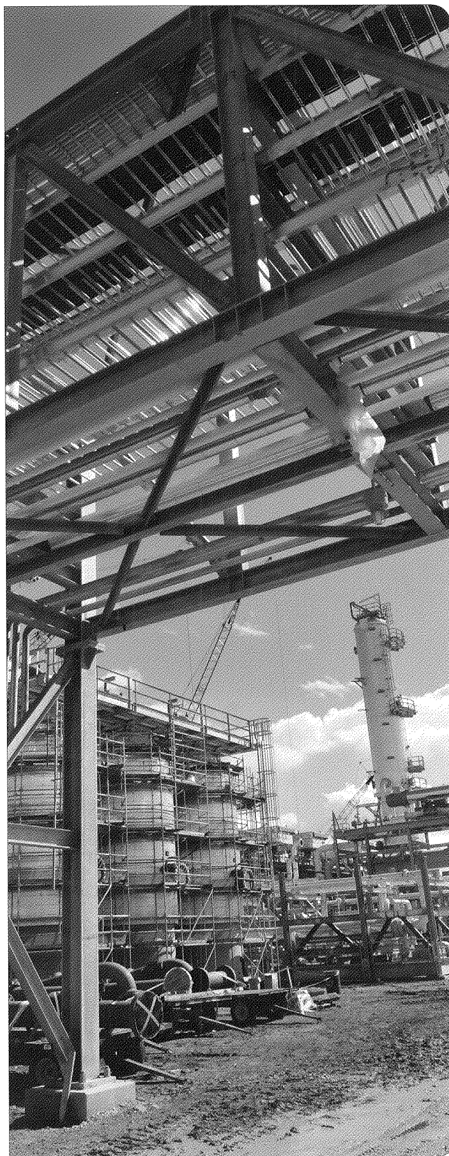
Century Plant pipe rack and absorber tower.
