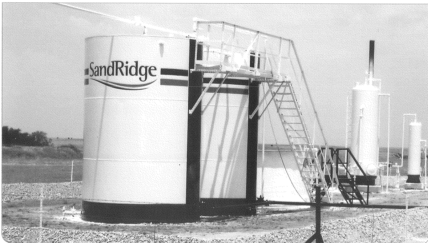
SandRidge tank battery.
