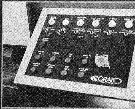
Access Control Point Electronic Security Controls.
