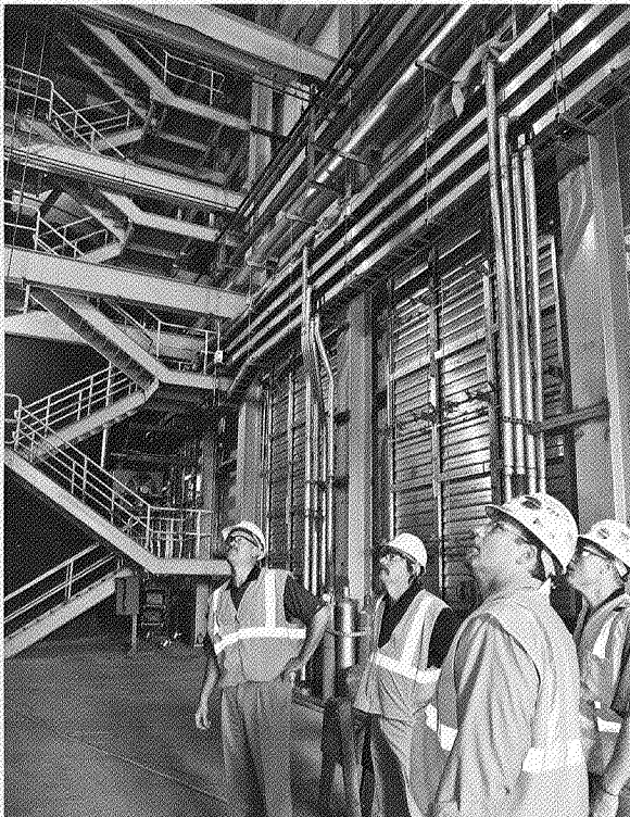
ALLETE President Al Hodnik, left, and others check out improvements at Boswell Unit 3, a major environmental retrofit completed in November of 2009.
