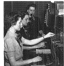
Left to right are Misses Hopkins, Berry, and Mariner, operators on the Richmond switchboard in 1943.
