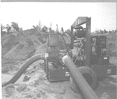
Prime Aire® pump used to dewater a holding pond at a sand quarry in North Carolina.
