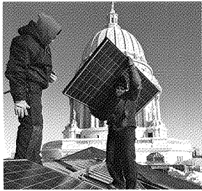
Workers install a set of solar panels on a wing of Wisconsin's state Capitol.
