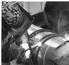
Brad Gordon, an MGE pipe-fitter, welds a steel gas main during a recent project.
