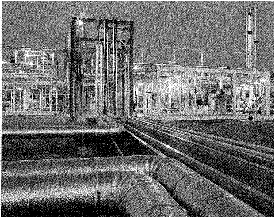
Our Henderson natural gas processing plant, located in Henderson, Texas, is part of our East Texas System. Both a cryogenic processing plant and a propane refrigeration plant are components of the facility.
