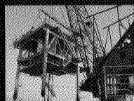
Offshore Services - 800-ton Arapaho Derrick Barge Decommissioning Maritech's Main Pass 181A Platform
