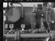
Production Testing - 1,440 psi High Pressure Three-Phase Test Separator
