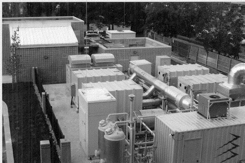
2.2 MW DFC-ERG in Toronto, Canada
