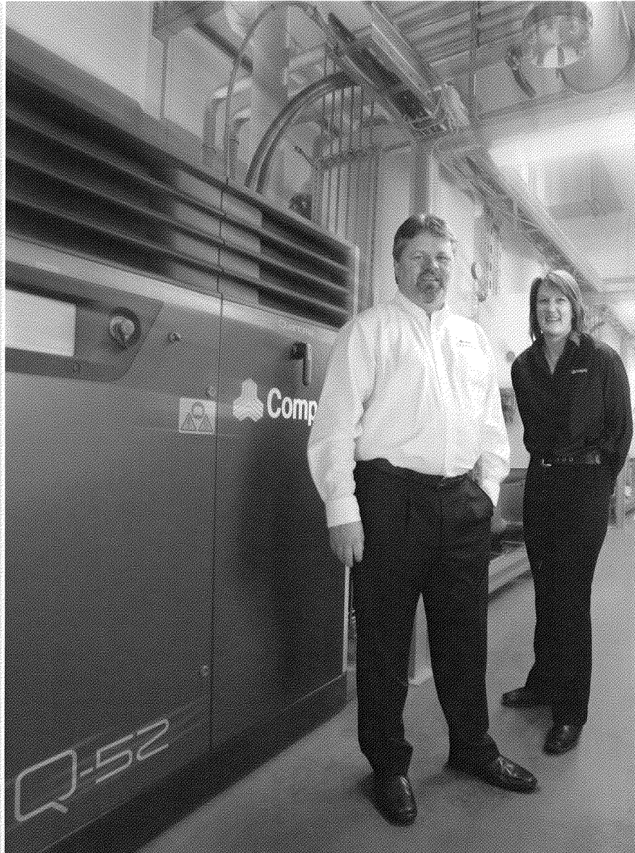
Jouko Peussa, Jassy Pyke and Kai-Arndt Doth of CompAir visiting a Quantima customer installation in Germany.
