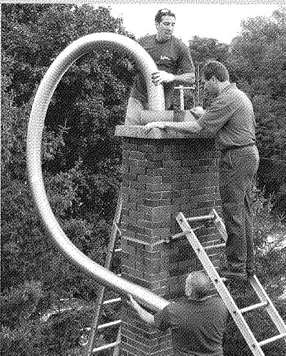
Simpson Dura-Vent®, Albany, goes into the field for a Ventinox installation. Chris and John from the Chimney Wizards and Jim Molloy, SDV Albany, holding on tight
