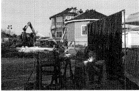
ABC-TV's "Extreme Makeover: Home Edition" design team selected Lincoln Electric as the show's exclusive welding partner. Pictured above is long-time show volunteer Jim Bollinger welding at a build last year in New Orleans.
