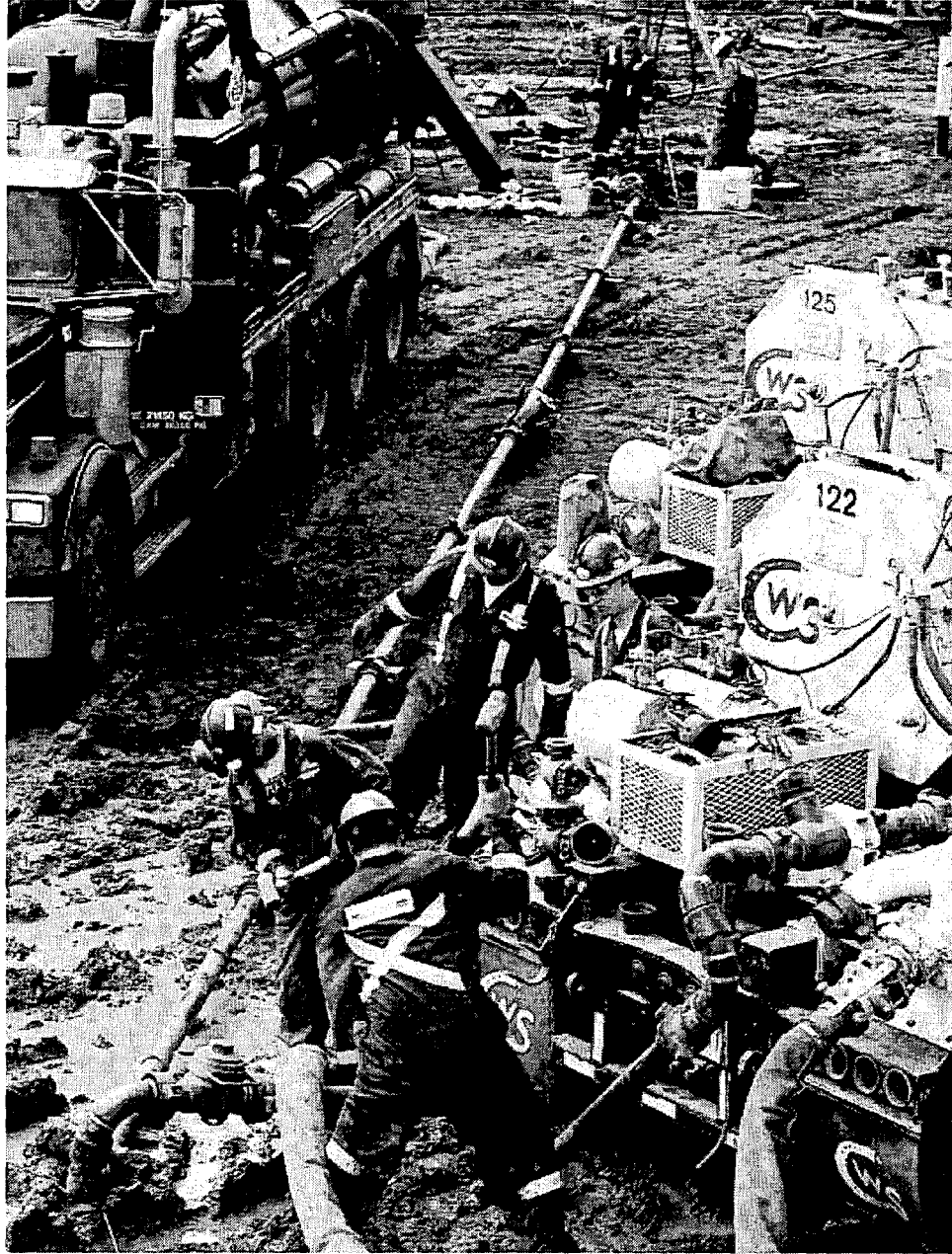
~ A treatment line is assembled in preparation of a high rate nitrogen fracturing job. The treatment lines are inspected regularly throughout the project to ensure wellsite safety is maintained.
