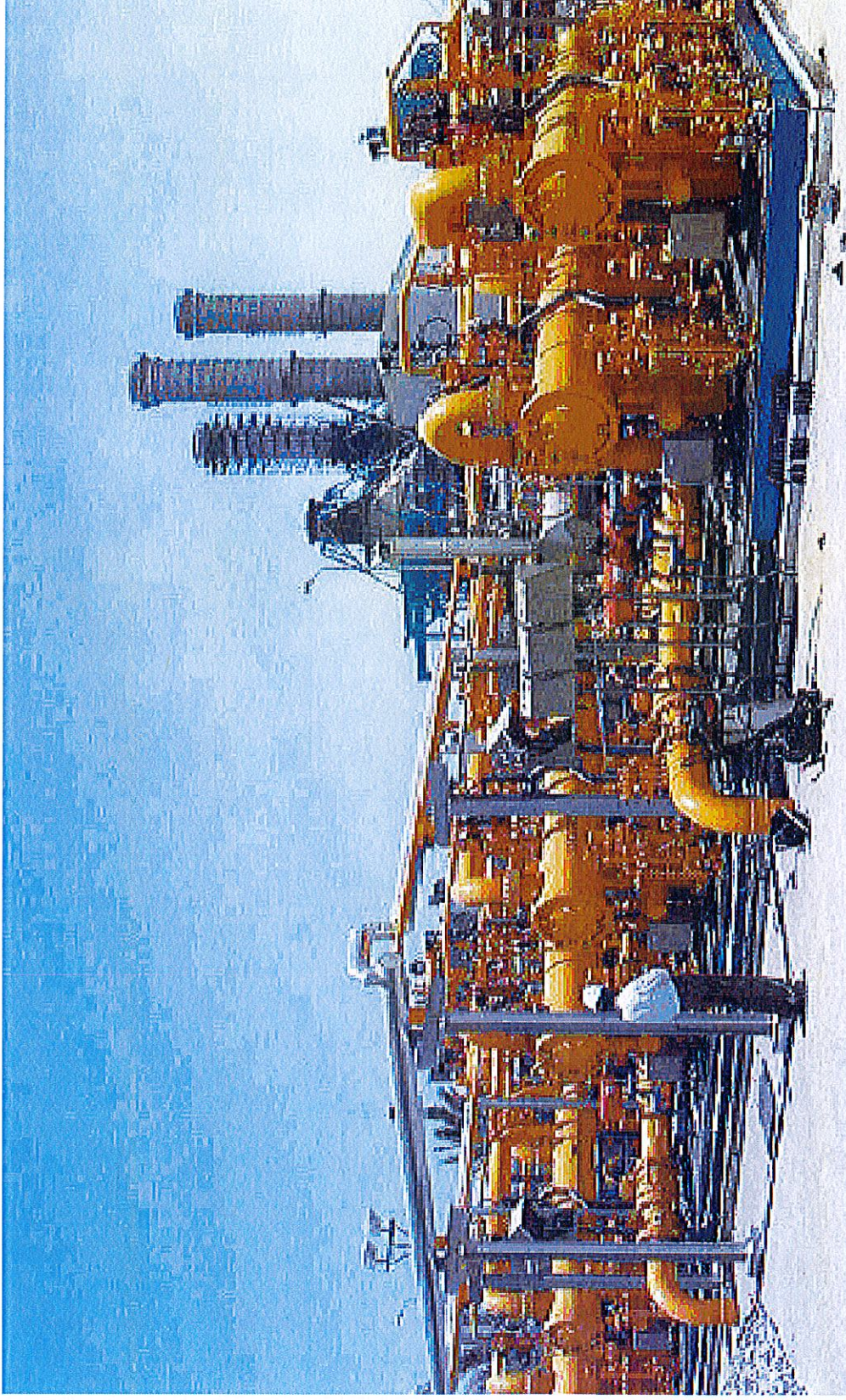
Fuel Gas Treatment System Jebel Ali Power Station
