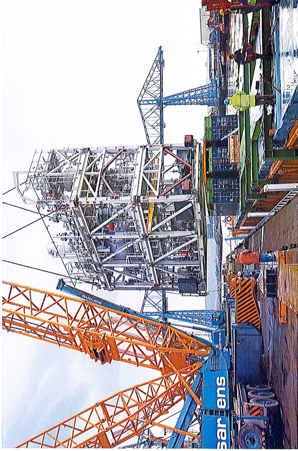
TEG Gas Dehydration Module for Gjoa Field in the North Sea
