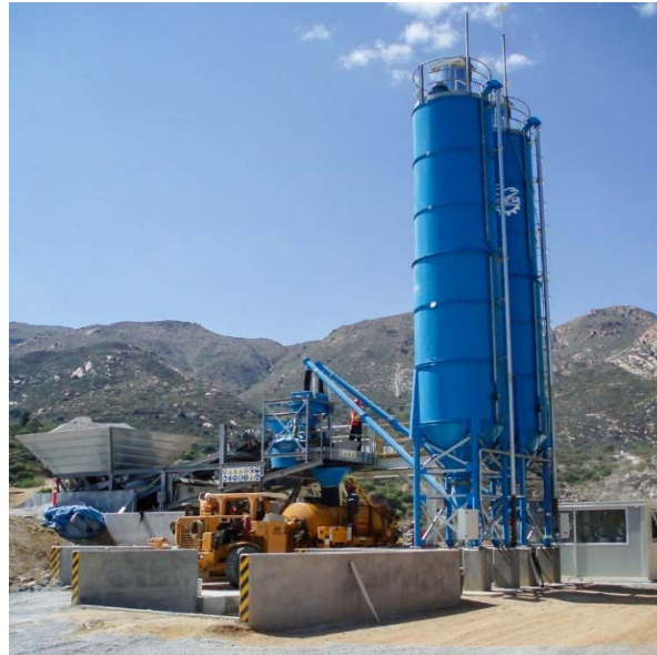
Figure 18-2: Concrete Batch Plant (Example)
