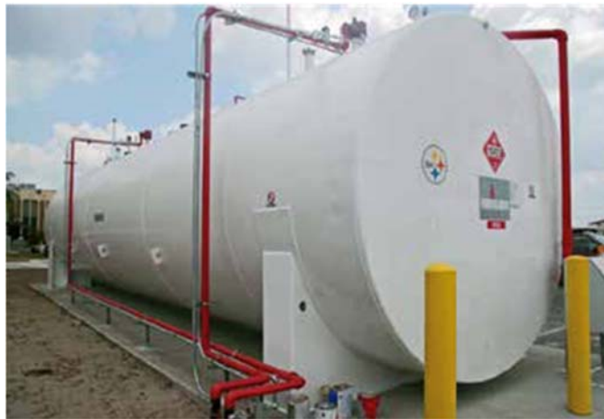
Figure 18-1: Aboveground Storage Tanks (ASTs) (Example)
