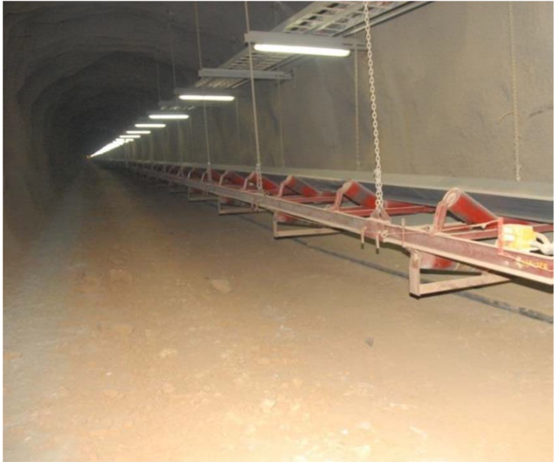
Figure 16-5: Typical Underground Suspended Conveyor Structure
