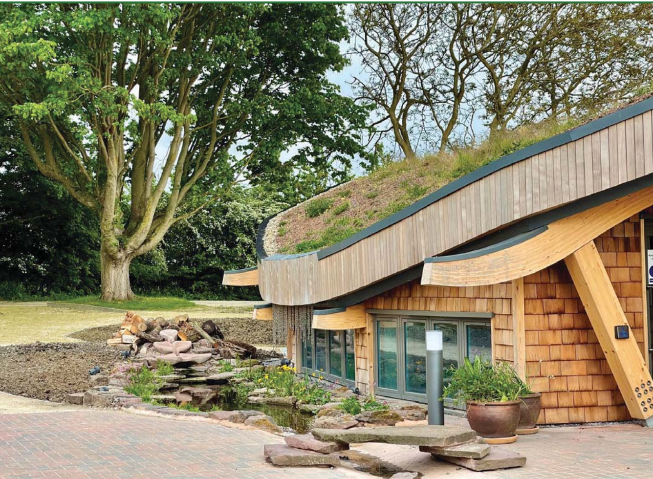
The Earth Trust's curved green roof was made watertight with RESITRIX hybrid EPDM membranes
