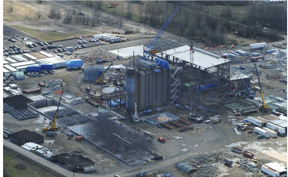
400 MW Port Westward plant (above) is expected to come online in Q1 2007.
