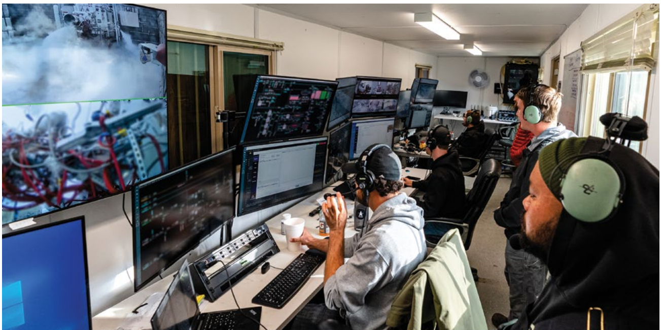
Control room at Astra's engine testing facility
