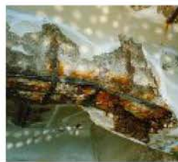
Sea Water Damage
