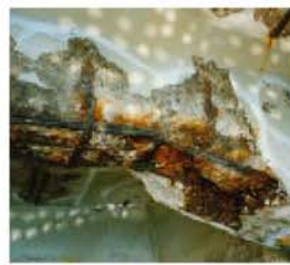
Sea Water Damage
