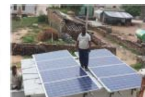
Shelter Top Solar Panels
