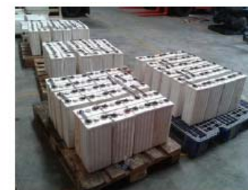
Release battery banks
