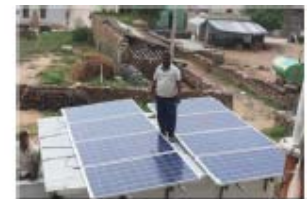
Shelter Top Solar Panels
