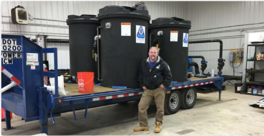
IX water portable demonstration units (1/5th scale)
