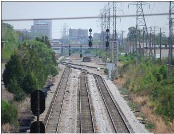
Poor Track on Passenger Line South of Acca Yard in Richmond
