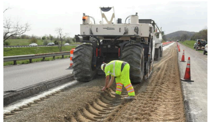
Work Continues on I-81 Pavement Recycling Project Courtesy of Virginia Department of Transportation
