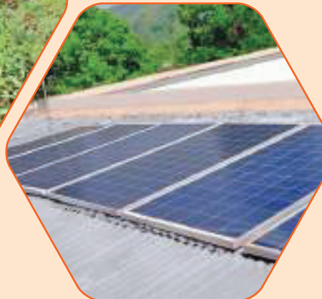
Solar panel installation in a school at Mawbri village in Ribhoi district, Meghalaya.
