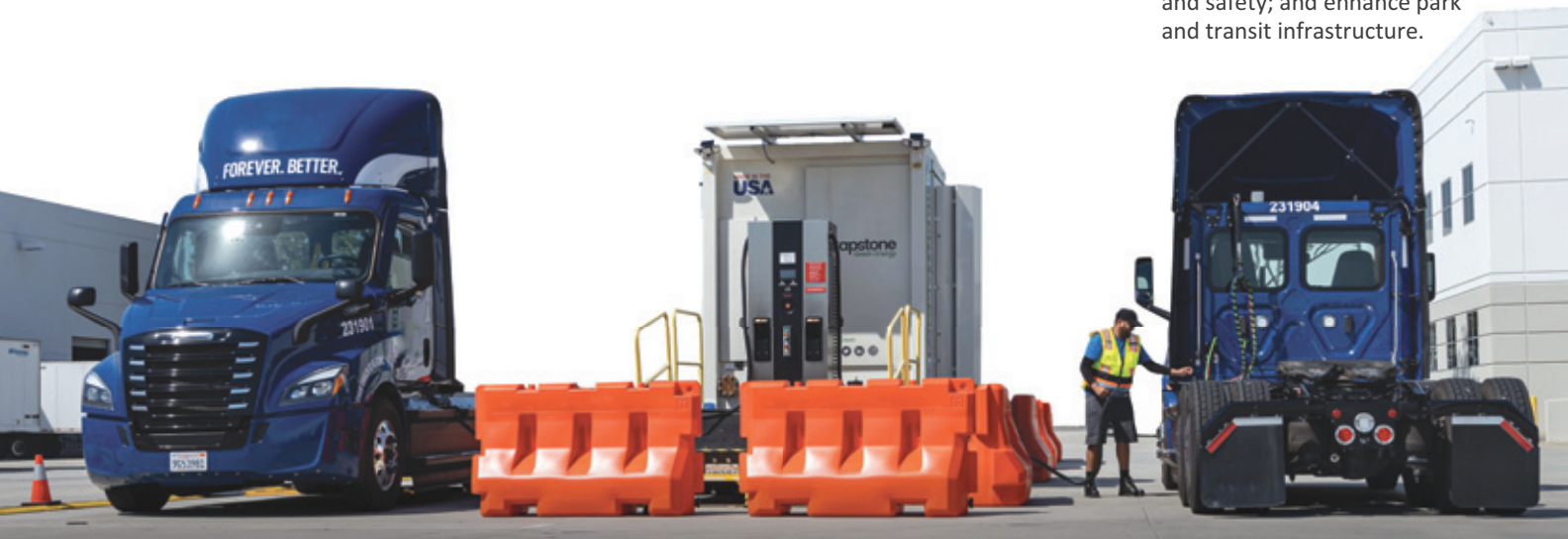
A temporary electric vehicle charging station at Prologis Torrance 1 property in Commerce, California.
