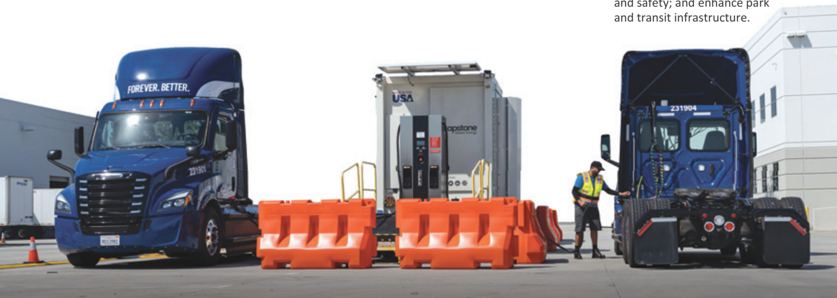
A temporary electric vehicle charging station at Prologis Torrance 1 property in Commerce, California.
